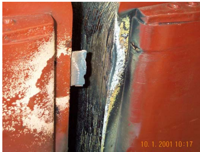
Fig. 2. Failed Lead Connector
